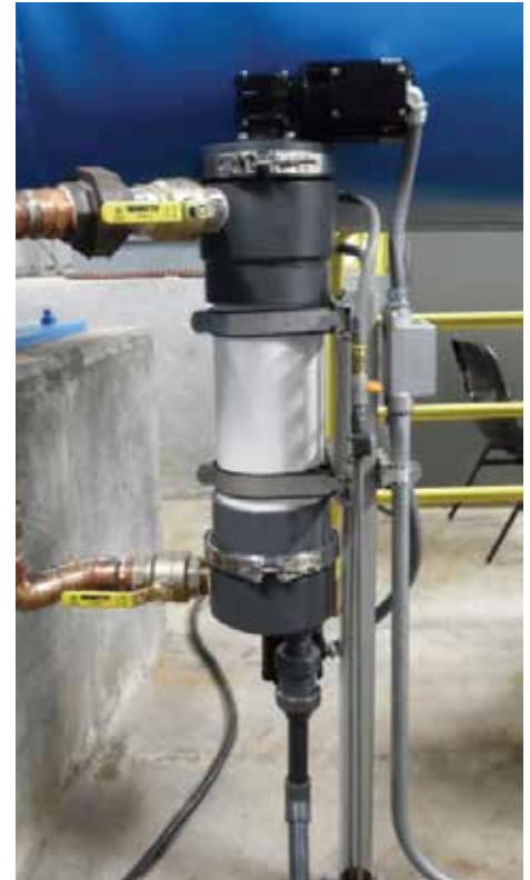
5: The 50-micron Spiral Water filter after installation
