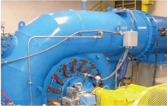
1: The hydroelectric turbine at the hydroelectric plant
