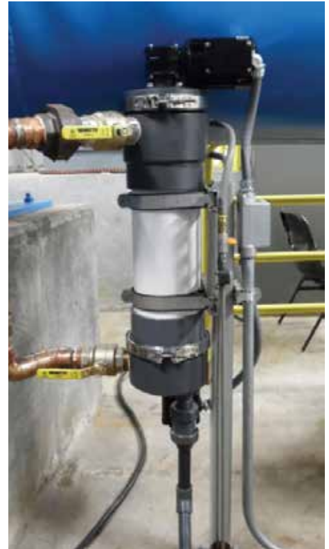
5: The 50-micron Spiral Water filter after installation
